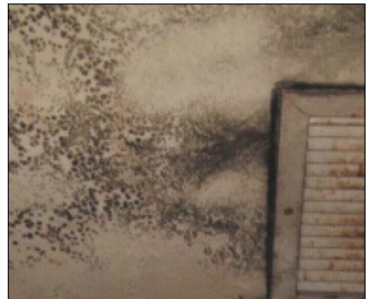
Mold growth adjacent to a ceiling vent.
